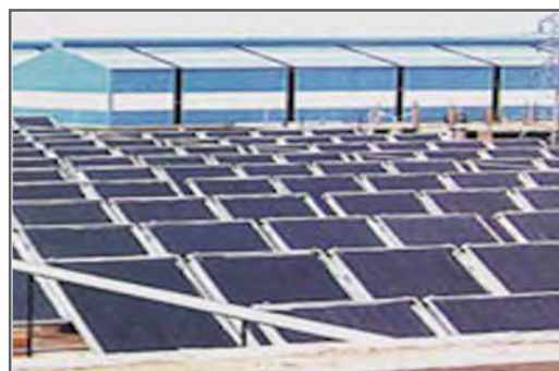
Fig 3.15: Solar Panels to trap solar energy
