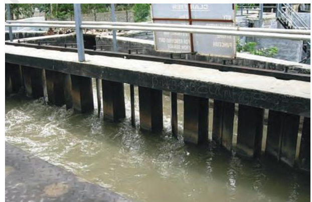
Fig. 18.4 Grit and sand removal tank
